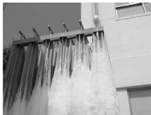
Fig. 4 Actual photograph on frost deposit of the general vaporizer
